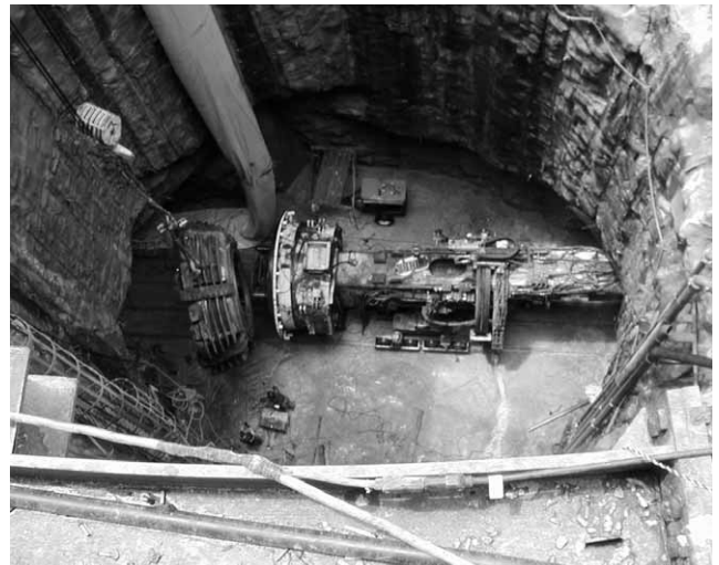
Bird's eye view of a tunnel-boring machine being used on the CSO project, Richmond
