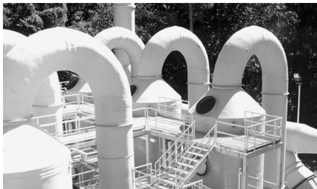
Odor-control scrubber towers at the Williamsburg Wastewater Treatment Plant. This is one of the three locations included in the HRSD odor-control project.
